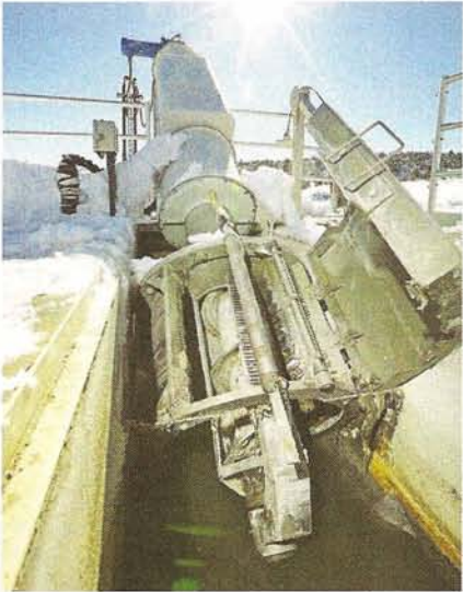
A Rotamat fine screen from Huber Technology does duty at the plant headworks. Large solids are captured on the screen, then washed off and deposited in a trash bin.
